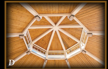
T & G subroof and no exposed conduit to interior lighting.
